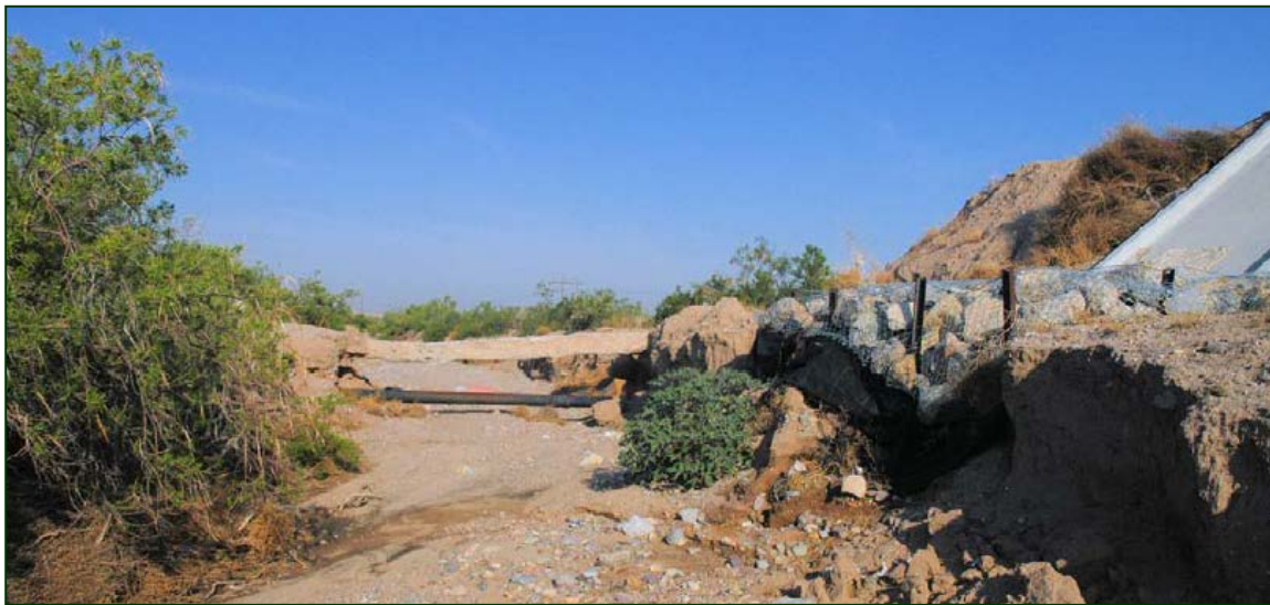
Exposed pipeline in an incised reach of the South Fork Arroyo downstream (west) from Roadrunner Parkway.
