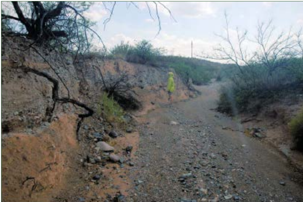
Looking downstream in typical portion of the incised reach of the Alameda Arroyo about 0.4 miles downstream from Alameda Dam where the left bank is being cut into an alluvial terrace. Photo: USACE Sediment Transport Analysis Report.
