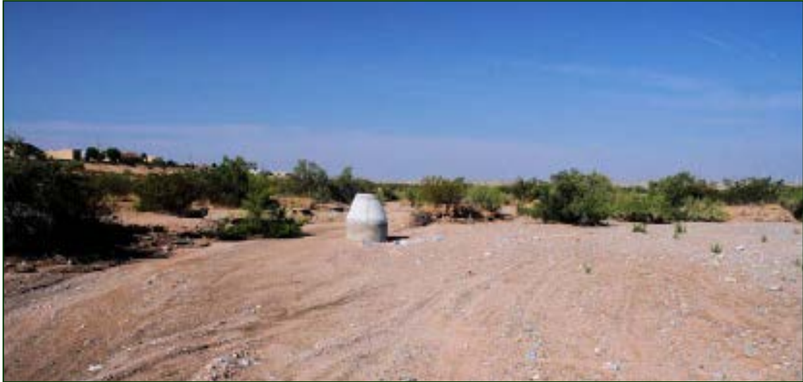
Exposure around the manhole indicates incision in this reach of up to 2 to 3 feet in this area. Note that some of the exposure could also be due to lateral movement of the low flow channel. This is the Alameda Arroyo looking downstream (west) from Roadrunner Parkway. Both photos: USACE Sediment Transport Analysis Report
