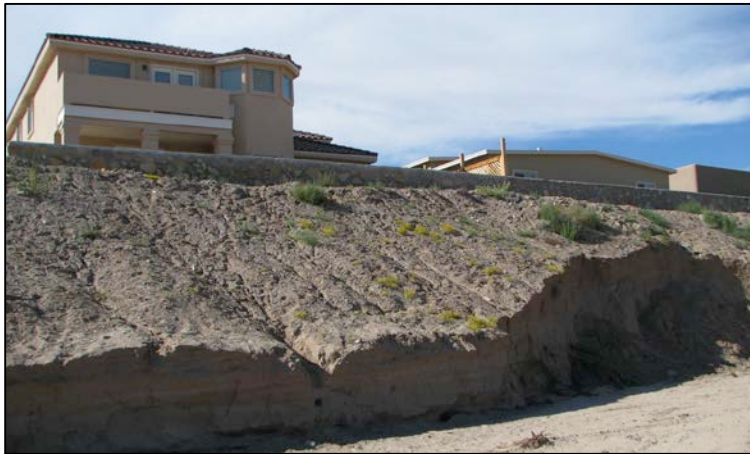
This photo illustrates what can happen when development restricts a natural channel. Continued erosion could eventually reach the point at which the retaining wall would have no support and would fall away. The photo below illustrates a quick and inexpensive (although unsightly) fix for the erosion problem. All photos: CLC Public Works Dept.
